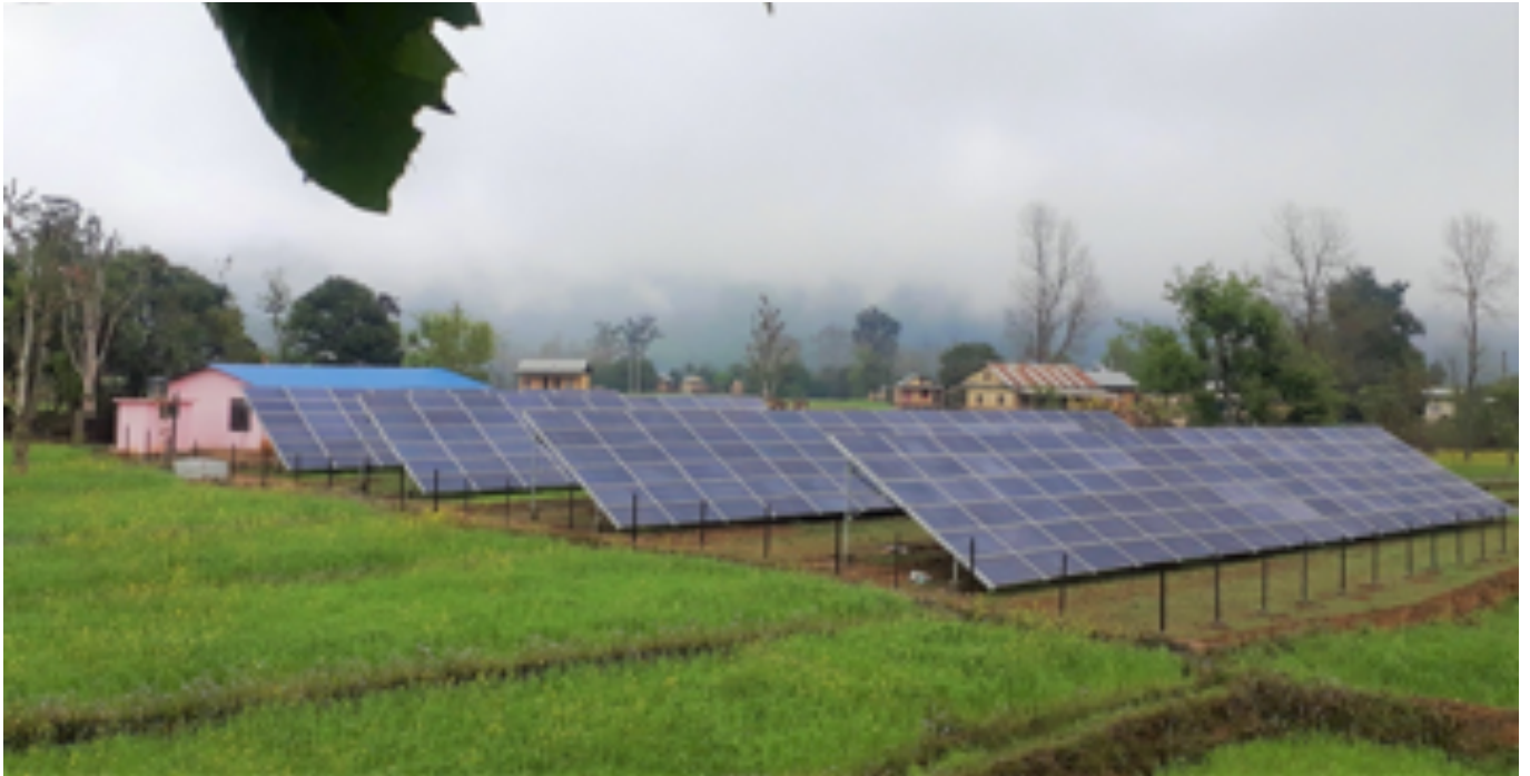
A mini-grid solar power plant with 100 kW capacity is installed located in the Gutu Village, Surkhet District, Nepal.
