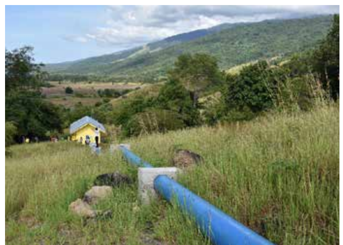
Micro hydro power plant installation with 100 kW capacity at Kawinda Toi Village located in Bima Regency, West Nusa Tenggara, Indonesia
