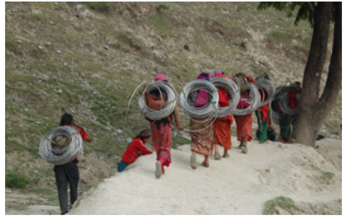
A group of rural women carrying transmission line of micro-hydro project for distribution system located in Gorkha District, Nepal
