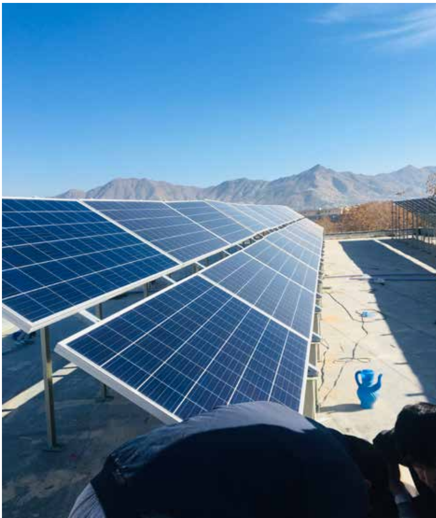
A solar rooftop project with the capacity of 20 kW is installed at the Training Centre of Ministry of Energy and Water of Afghanistan.
