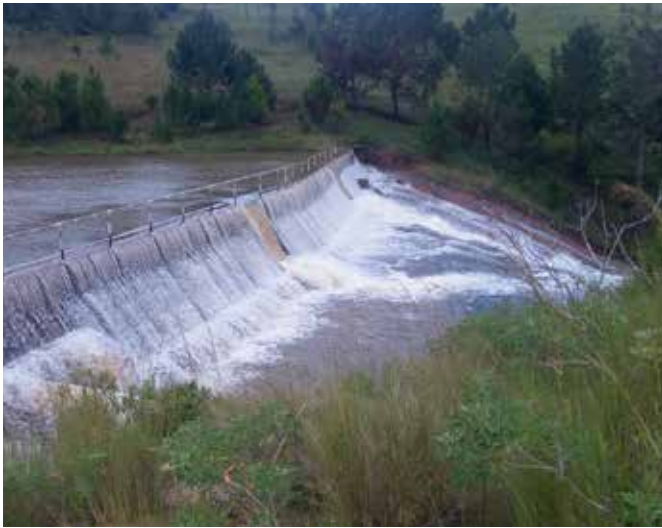
A hydroelectric site generating electricity with the capacity up to 60 kW at Soavina in the rural commune of Ilaka Centre, Madagascar. This site was developed with the support of technical and financial partners, including GIZ through PERER Program.
